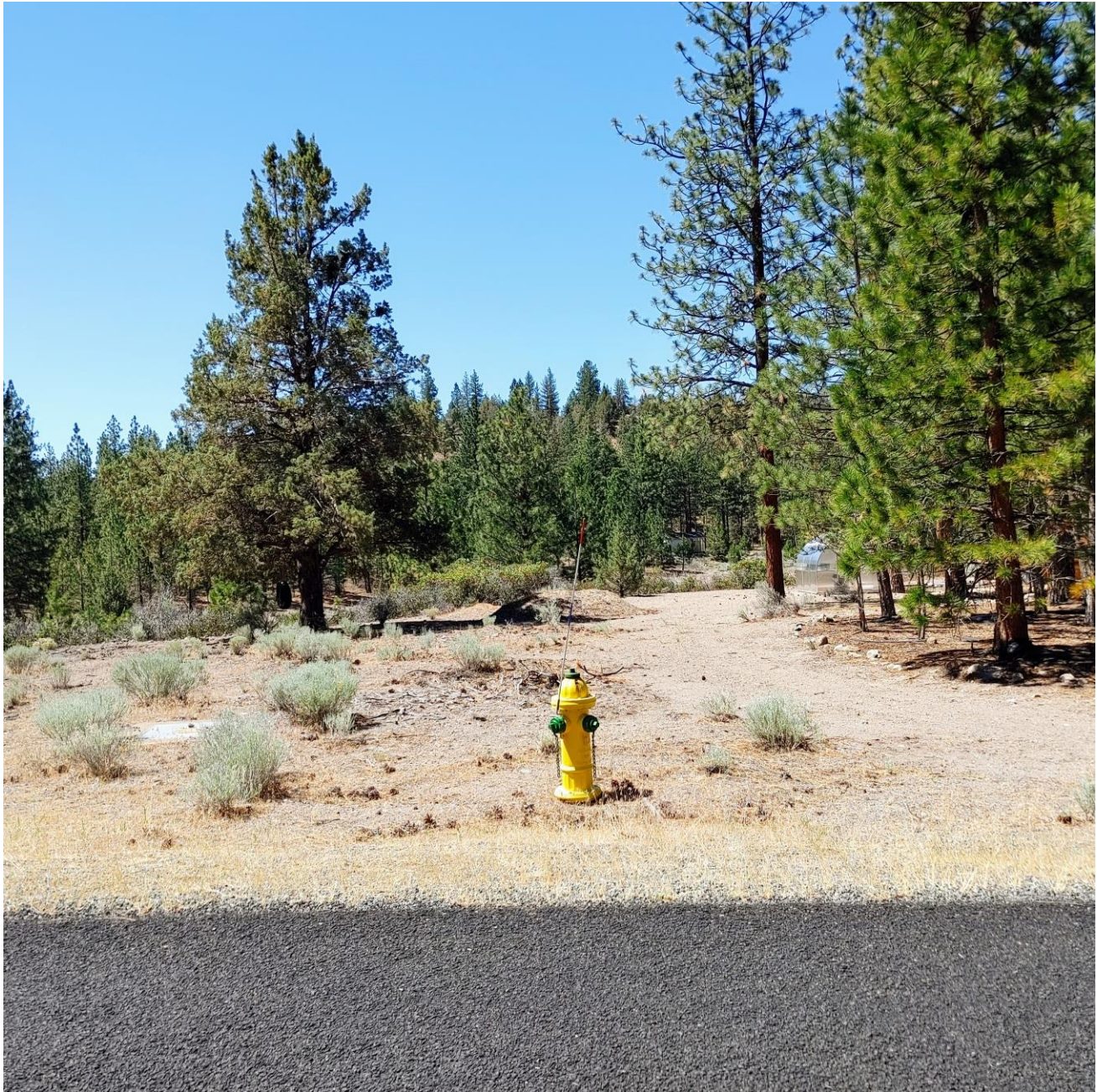
Photo 9: Looking south west from Indian Island onto fire hydrant #79 that will be replaced with a new fire hydrant. This fire hydrant is surrounded by small rabbit brush, gravelly soil, ponderosa pine, and juniper. The soil directly around the fire hydrant will be disturbed as all parts of the hydrant will be replaced down to the elbow in the ground.
