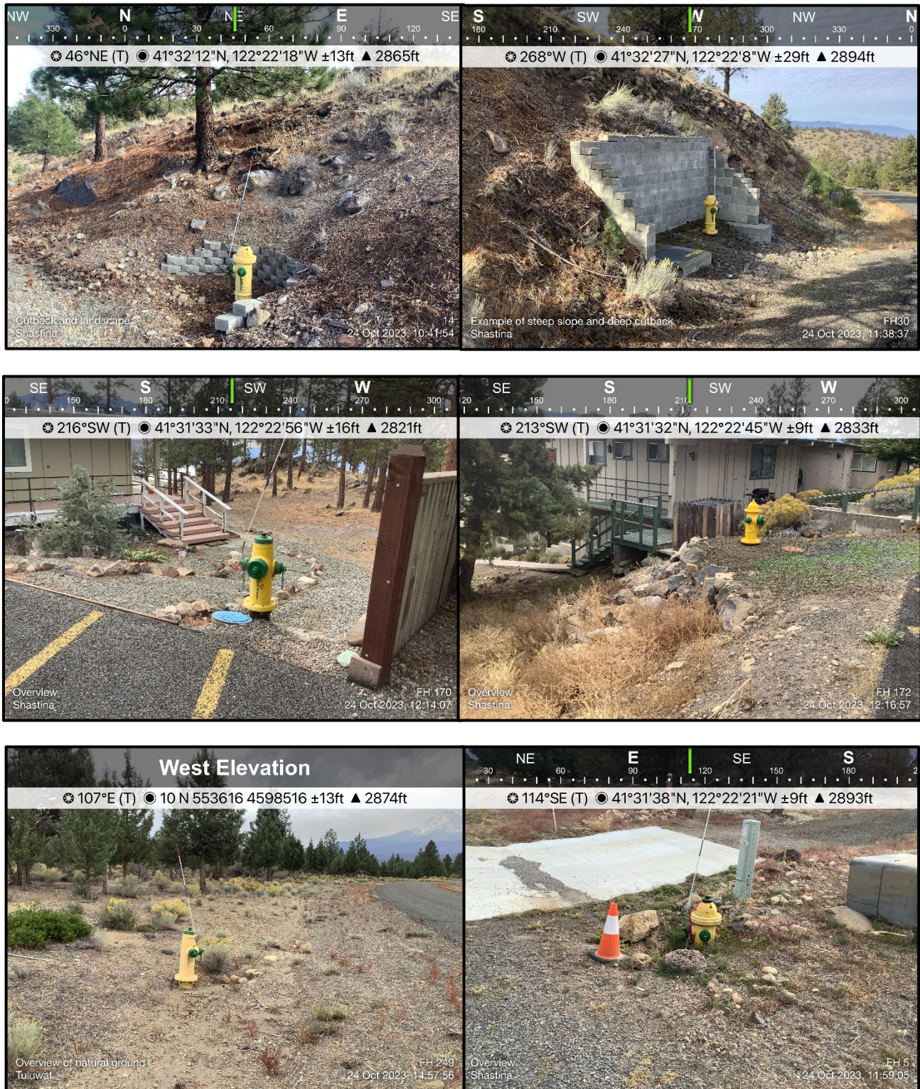
Figure 5. Range of typical fire hydrant installation conditions, ranging from highly developed & engineered landscaped installations (upper L and R), to highly modified natural landscapes (middle L & R), to moderately modified landscapes (lower L & R), all of which tie into the main system at the adjacent street curb.
