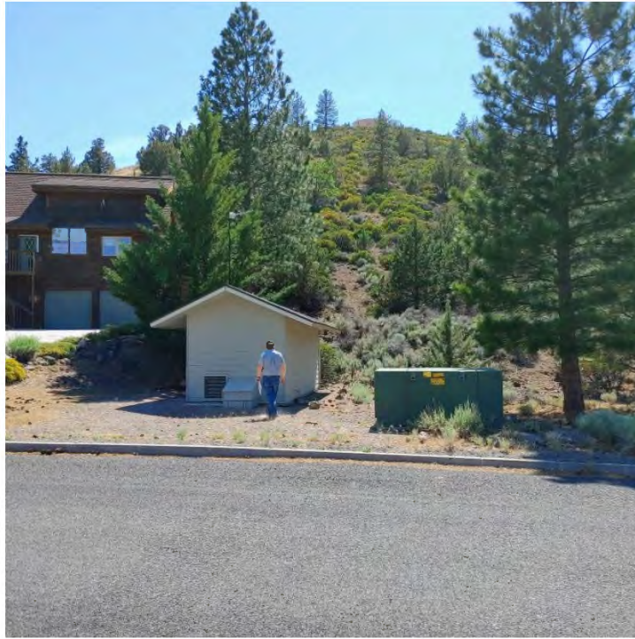
Photo 1: Looking west at pump station 53 on Palmer Drive where the location of the temporary water tank outside of the building would be placed as water tank 4 is upgraded to a bigger size. Water tank #4 can be seen on top of the slope. Gravel is observed on the east side of the pump station where the temporary water tank would be placed. Photo taken: 6/22/2022.
