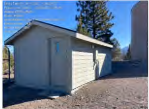
Photograph 3.9 Booster Pump Station B-51
