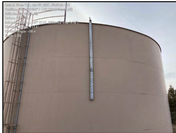
Photograph 3.4 Juniper Tank (Tank 1) showing manual tank level gauge.
