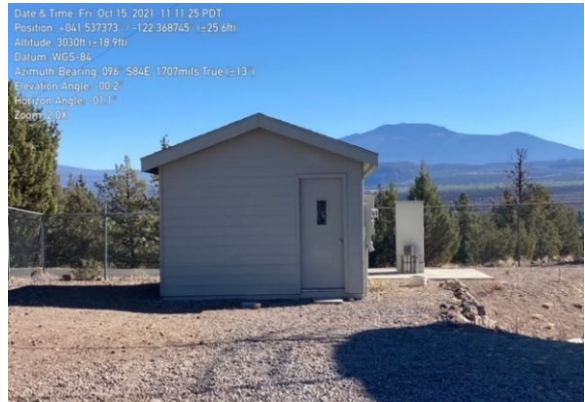
Photograph 3.8 Booster Pump Station B-50
