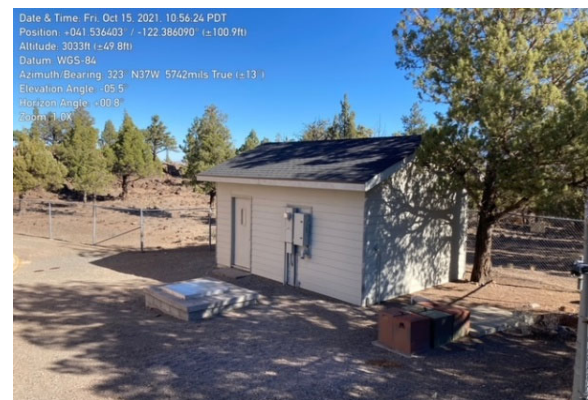
Photograph 3.10 Booster Pump Station B-56
