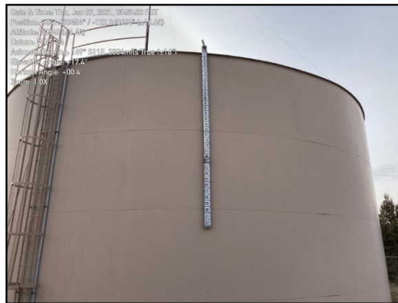
Photograph 3.4 Juniper Tank (Tank 1) showing manual tank level gauge.
